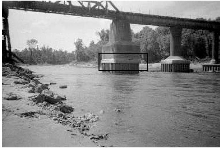
Fig. 8. Railroad bridge near Goodrich, TX between Livingston Dam and the Romayor gaging station. The box in mid-photo highlights a concrete pad that was flush with the river bed when the bridge was constructed in 1917. At the time of the photograph (May 2002), the pad was about 2 m above the water surface and 5 m above the channel bottom.
